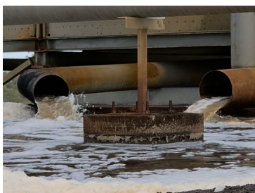
Cooling tower returns falling into the tank and entraining air.
