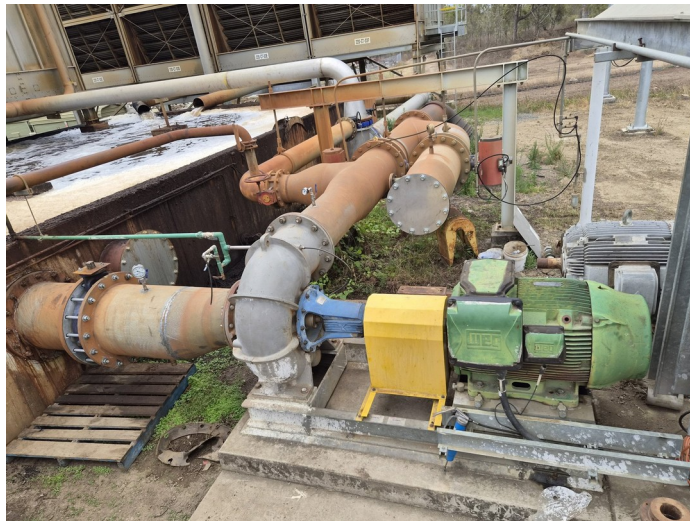
The injection cooling water pump set and suction arrangement from the cooling tower tank.
